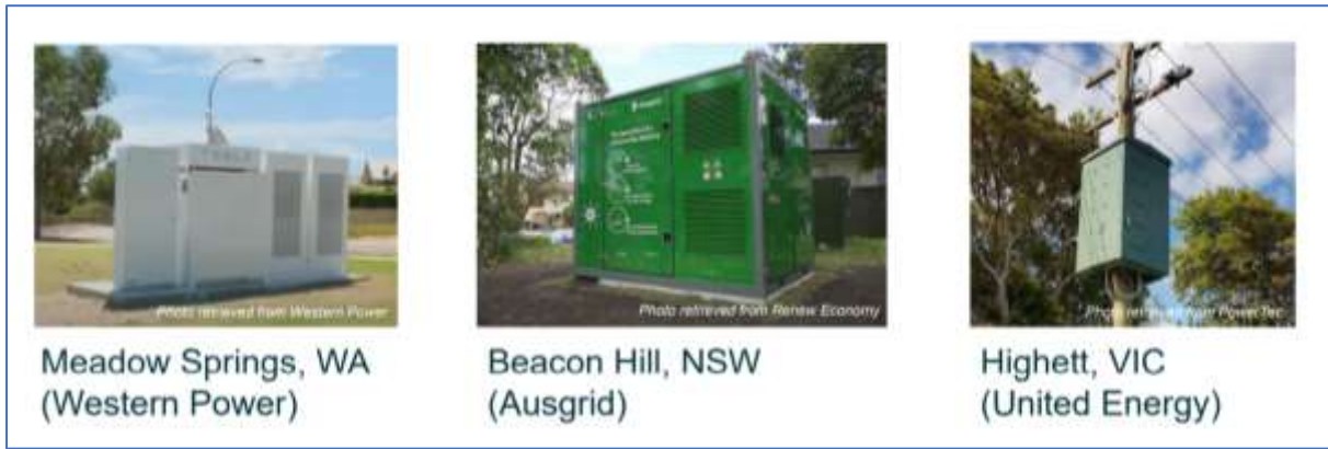
Figure 6 Pad and pole mounted Local Batteries
